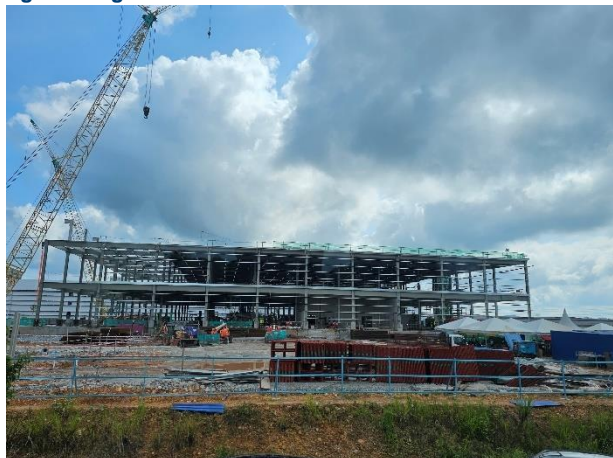
Fig 8: Bridge Data Centres site in STeP
